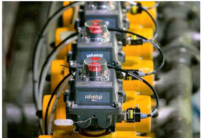
TopWorx Valvetop DXP discrete valve controllers installed at MAPEI plant in West Chicago, Illinois
